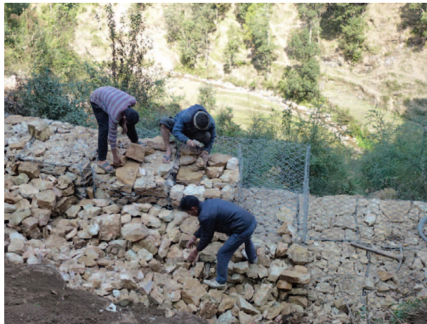
Photo 9: Packing the wire mesh properly is paramount for the stability of walls of gabion boxes
