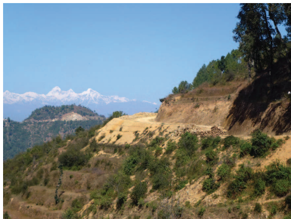
Photo 2: If applicable, roads along the ridge top should be preferred over valley bottom alignments
