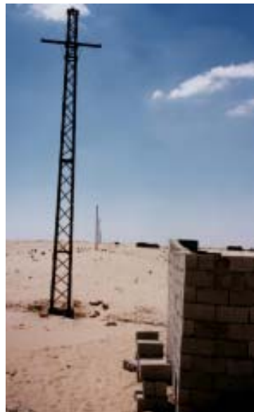
Photo 2: Electricity poles have been mounted and a chamber for the transformer (foreground) has been constructed
